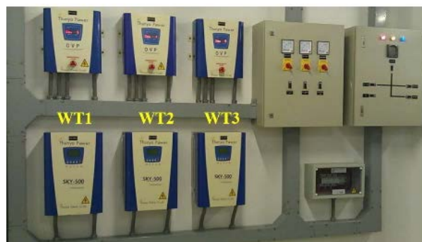
Fig. 13. Grid-connected inverters of THUNYA-5kW HAWTs in electrical control room of DETC.
