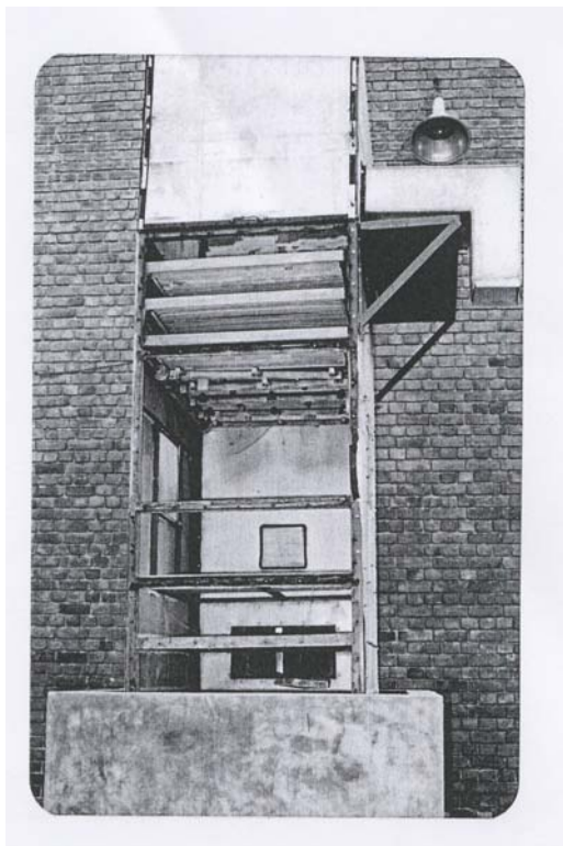
Fig. 2. Inside View of the Spray Filled Tower
