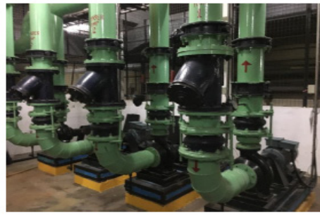
Existing Condenser Pumping System
