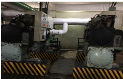
Existing Carrier 180 TR Water Cooled Screw Chillers
