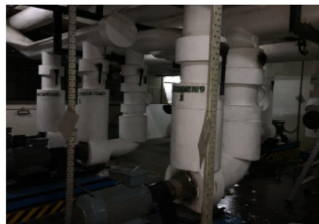
Existing Primary & Secondary pumping system
