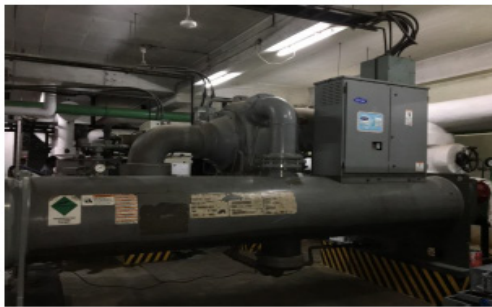
Existing Carrier 337 TR Water Cooled Centrifugal Chiller
