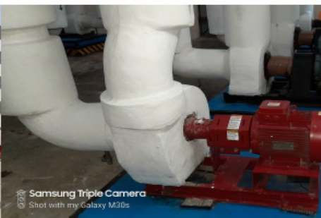
New High Efficiency Primary Pump
