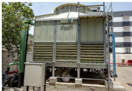
New High Efficiency Cooling Tower
