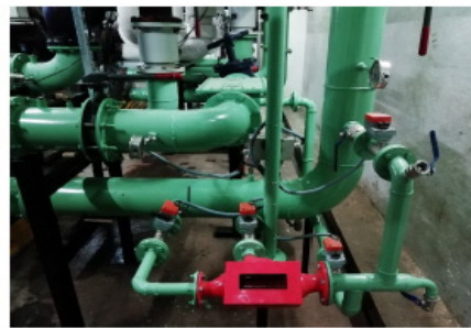
Automatic Tube Cleaning System (ATCS)
