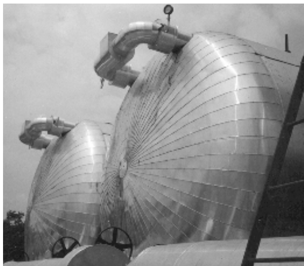
Fig. 5. Photographic view of cool thermal energy storage tanks.
